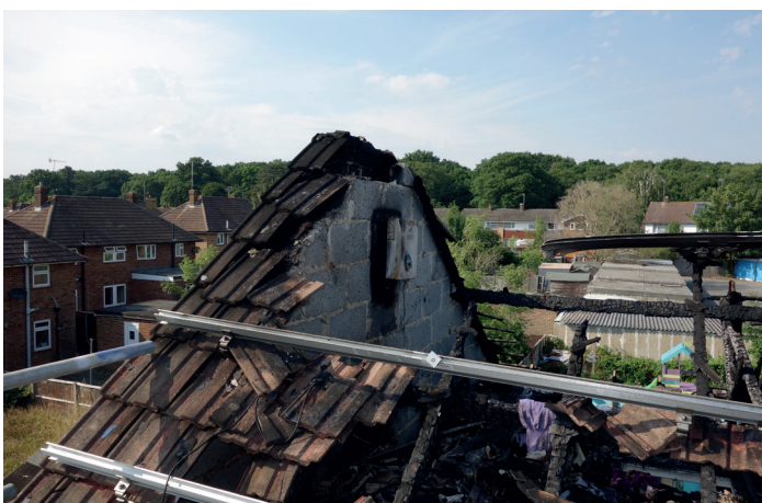
Figure 22: Damage to a roof resulting from a fire in a PV system
