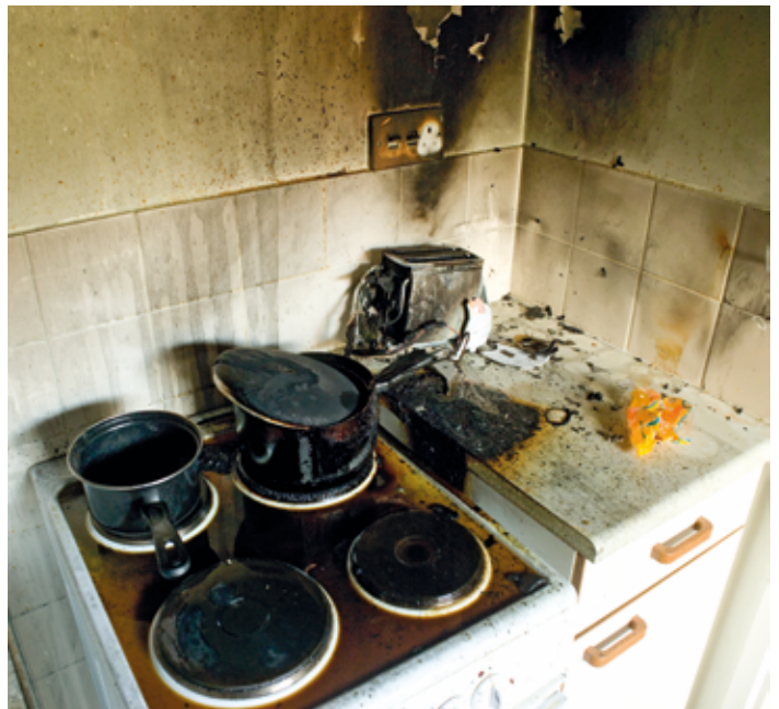
Figure 14: Heat alarms can detect and provide warning of fires in kitchens
