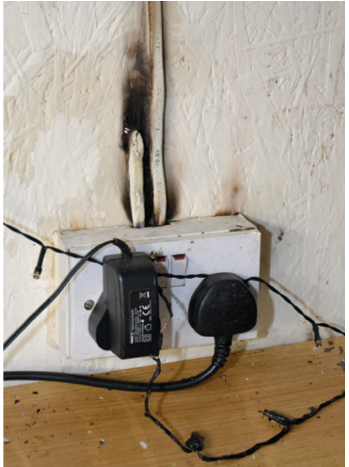
Figure 4: Example of a fire due to an electrical cause (photo courtesy of SFRS)
