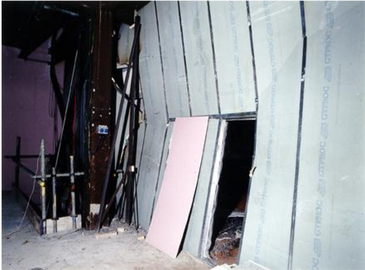
Photograph 11 Deformation of compartment wall – view from outside compartment
