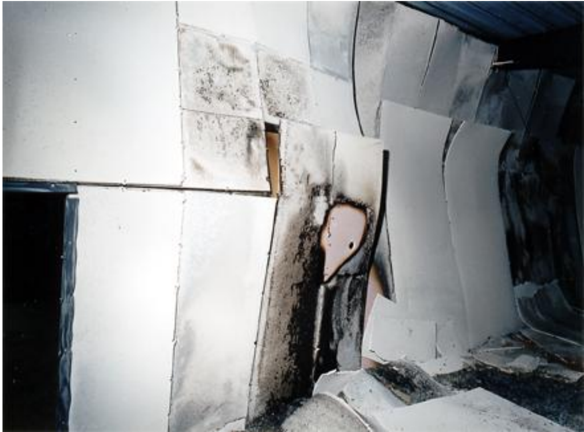
Photograph 10 Localised collapse of compartment wall – view from inside compartment
