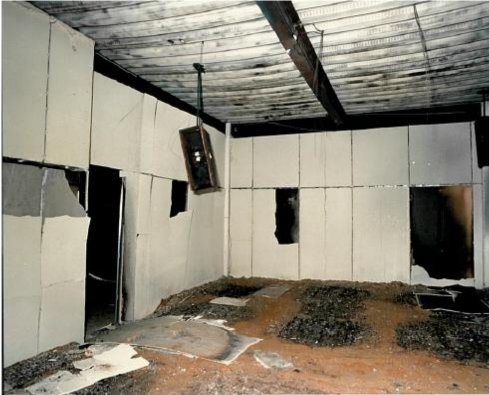
Photograph 5 Corner fire compartment post-test
