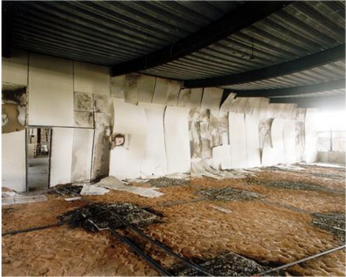
Photograph 9 Deformation and integrity failure of compartment wall – view from inside compartment
